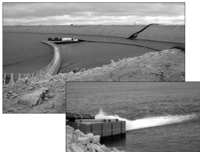
With the successful airlift of construction supplies, Diavik's new 1.3 kilometre A418 dike construction is on schedule. In September dewatering was progressing as planned with clean, clear water being pumped into Lac de Gras.
