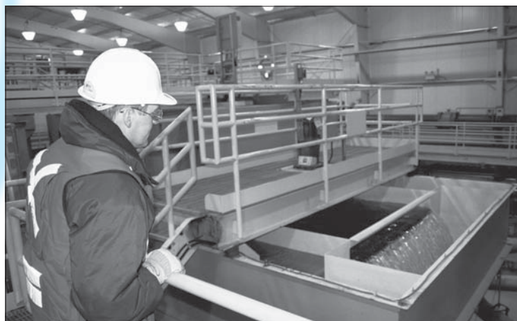
Diavik's water treatment plant is successfully treating muddy waters created and then stored during last year's dike dredging program.
